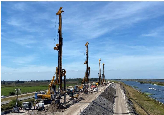
Figure 6: Two RTG RG 27S (front) installing CSM cutoff wall in perpendicular mode at TO1 east.
