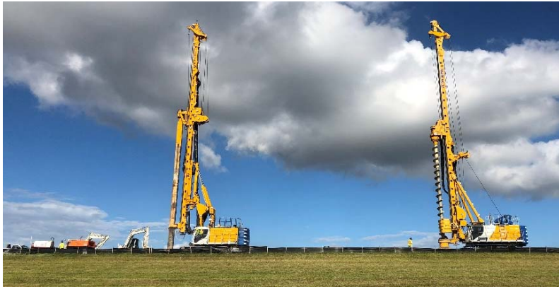
Figure 4: Bauer BG 30 drill rig performing CFA predrilling (right) and RTG RG 27S installing CSM cutoff wall (left) at TO3 west.
