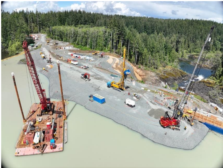
(2) For safeguarding work on the dam, a BAUER BG 30 was used for this soil improvement work along with other equipment.
