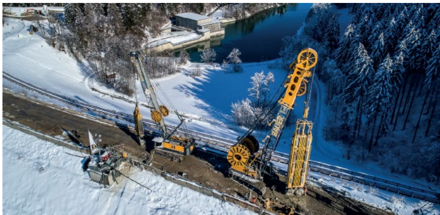
Fig. 12. BAUER MC 96 with turnable BAUER HDS-T hose reel system and BC 40 trench cutter (right) BAUER MC 64 equipped with BAUER DHG hydraulic grab
