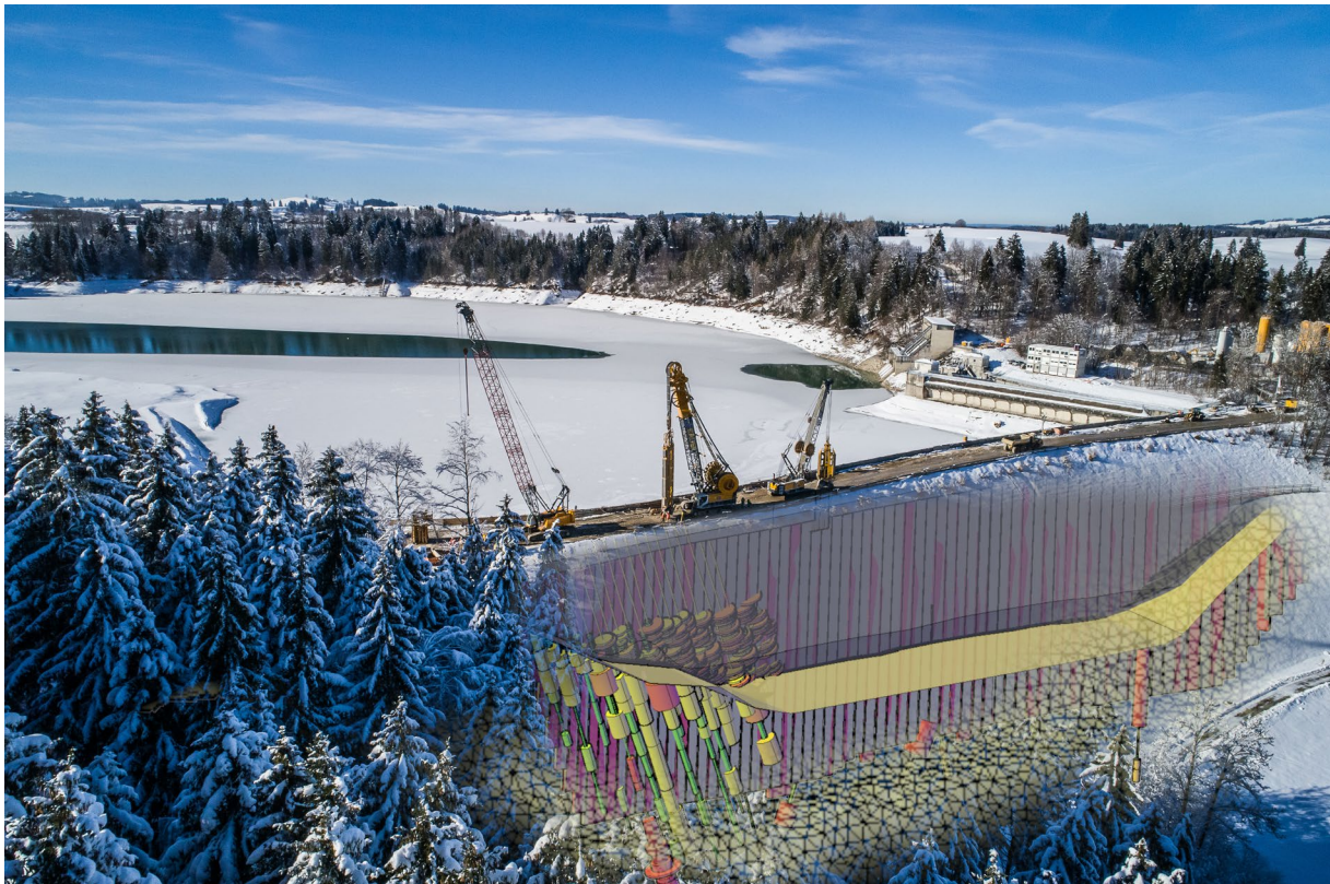
Fig. 18. Photo showing both the execution of cut-off wall in winter, and the results of the Quality Control
