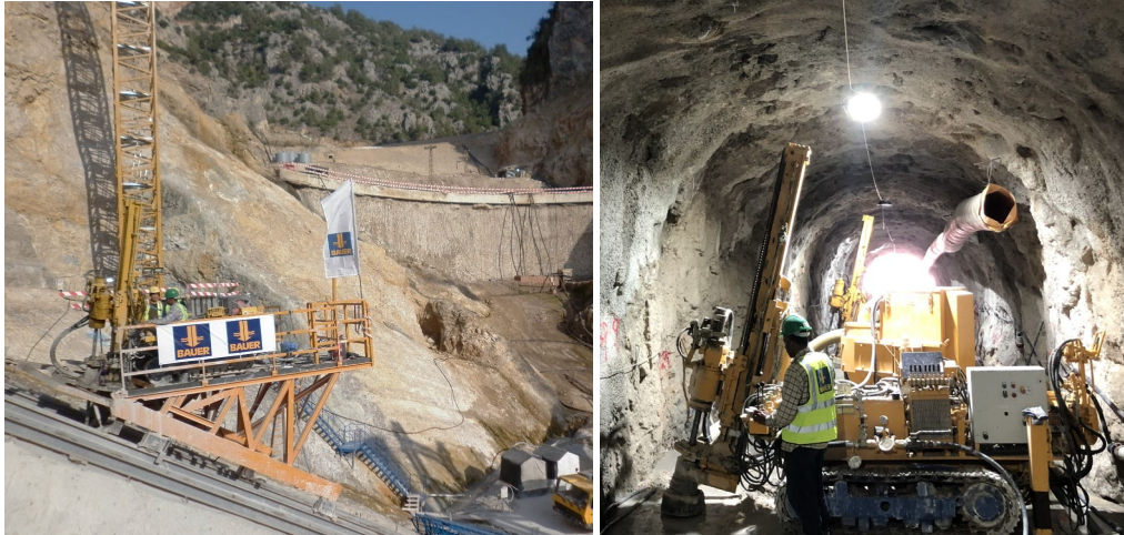
Fig. 12 Mobile platforms on special rails for drilling and grouting works on slopes, exposed bulkhead in the background (left) [1], and working in galleries using electrical drilling rig (right)
