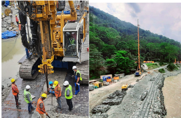
Fig. 6. Redrilling for jet grouting and predrilling of the holes in the boulder strata along the alignment
