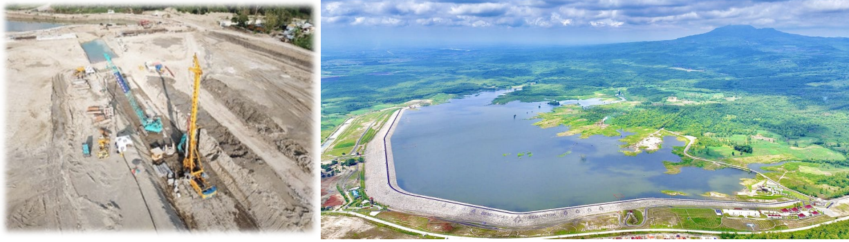
Fig. 2. Execution of secant pile wall (left), and picture showing the current status of the project
