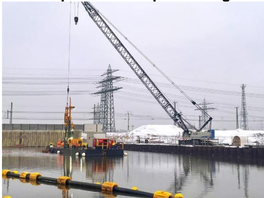
(1) West trough pit for future tunnel below the dam of the harbor railway
