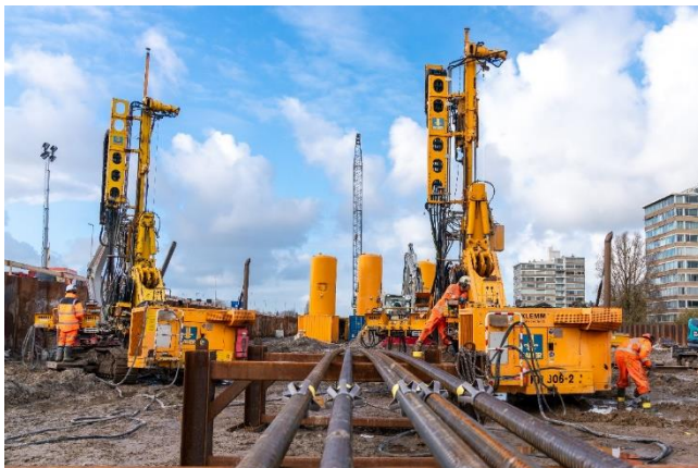
(2) A total of approx. 12,000 anchor piles will be drilled to an average depth of 33 m along a 1.7 km section of the highway.
