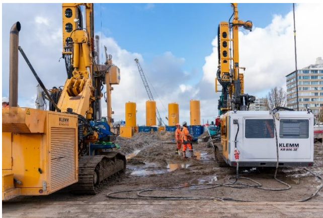
(1) First use of the newly developed KR 806-3E electric drill from KLEMM Bohrtechnik GmbH on a construction site in Amstelveen
