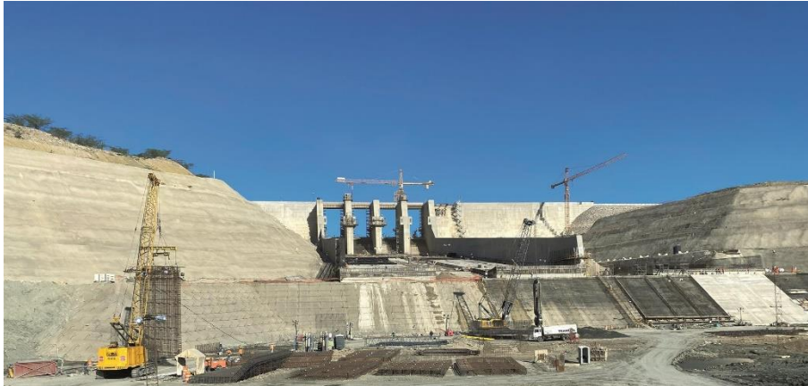
(1) From May 2022 to March 2023, Bauer constructed a total of 55 diaphragm wall panels.
