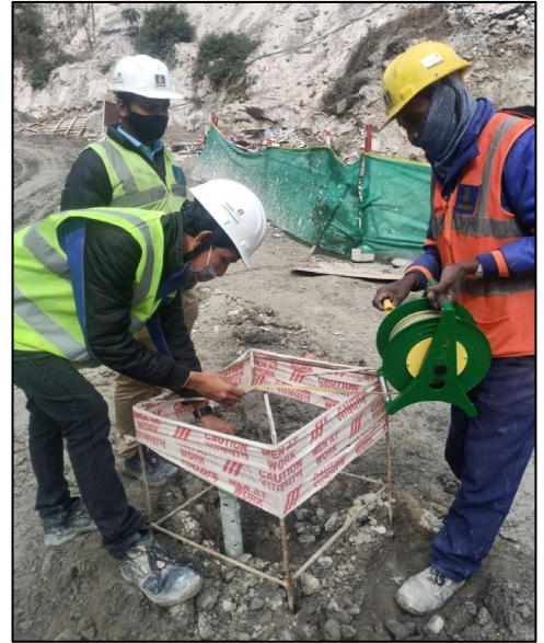
Figs. 5. Observation of GWT in observation bore hole with water detecting sensor
