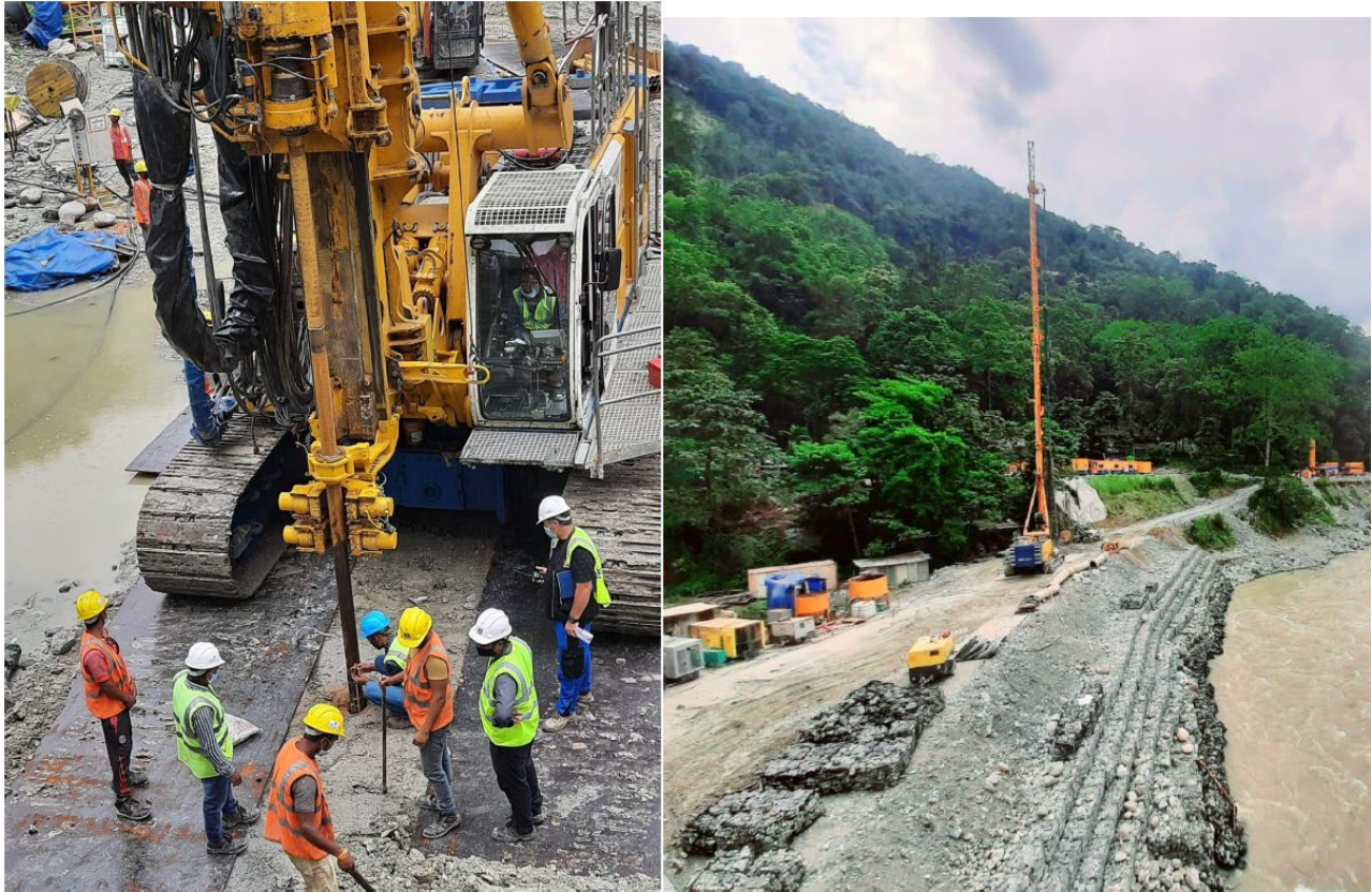
Fig. 10 Redrilling for Jet Grouting and Predrilling of the Holes in the Boulder Strata along the alignment
