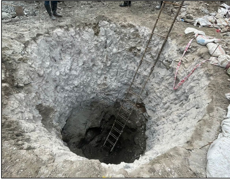
Fig. 4. Visual Inspection of Seepage
