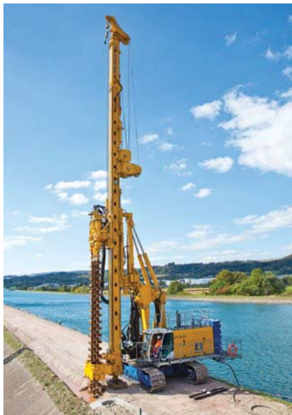
Figure 4: Manufacturing of the Mixed-in-Place cut-off using a RTG RG 25 rig with a triple auger
