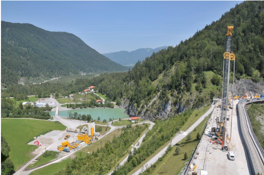
Fig. 7: Construction Tasks – narrow platform width and permanent traffic upstream along the platform
