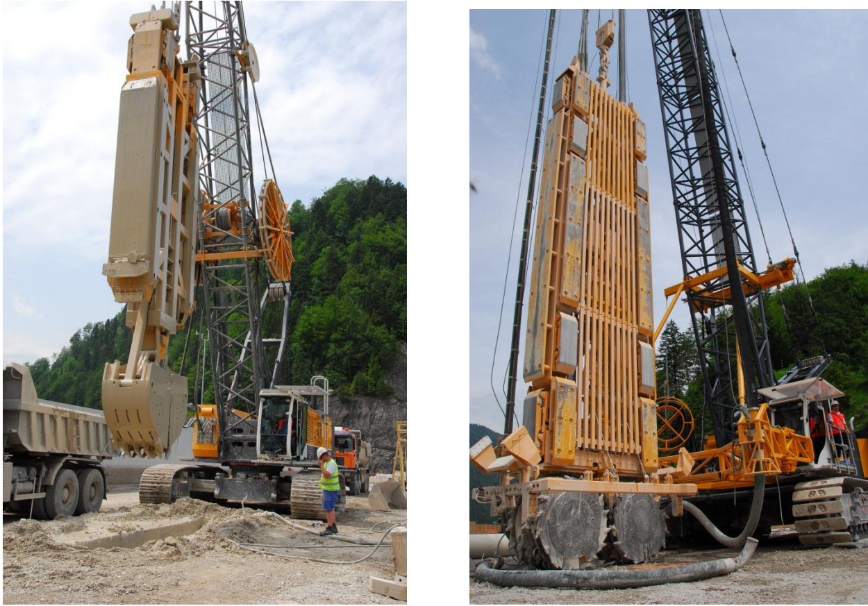
Fig. 5: The main equipment; left: BAUER MC 64 with hydraulic grab – right: BAUER MC 128 wit BC 40 Cutter
