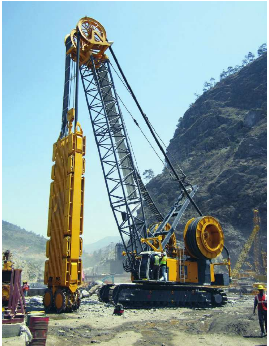
BAUER MC 128 Base machine with HDS and Trench Cutter BC 40 rigged up for rock cutting to depths of more than 100 m (328 ft) (© BAUER)
