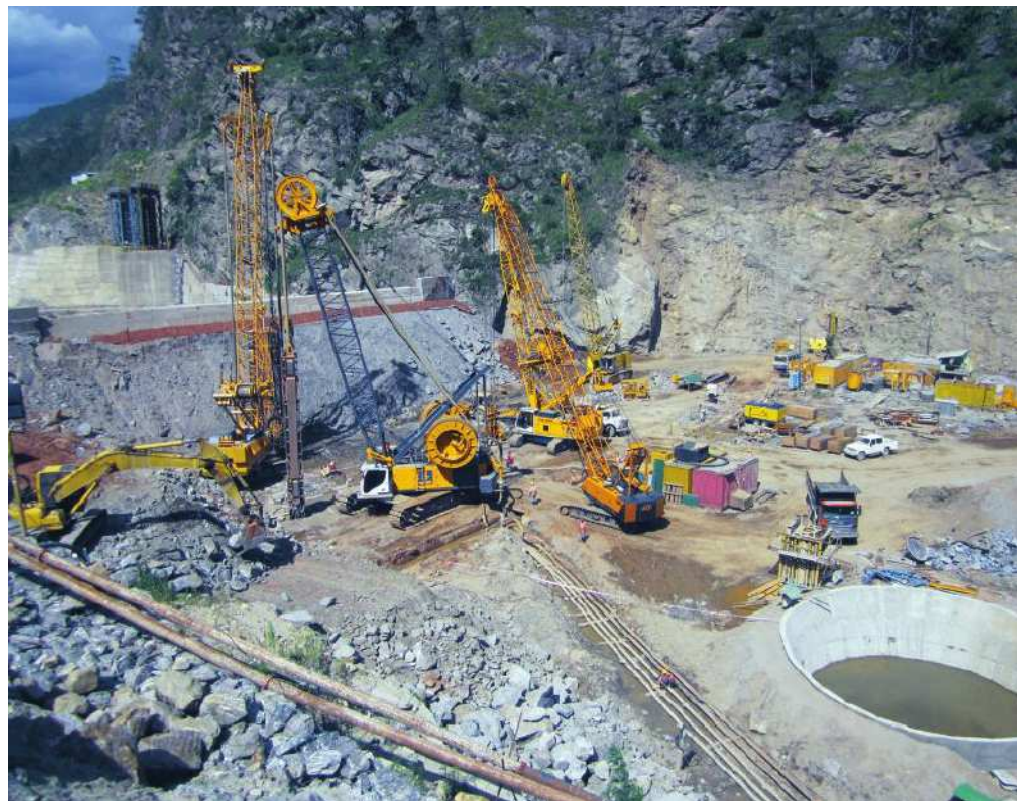
The concrete cut-off wall with two BAUER Trench Cutters, one BAUER Hydraulic Grab and support cranes (© BAUER)
